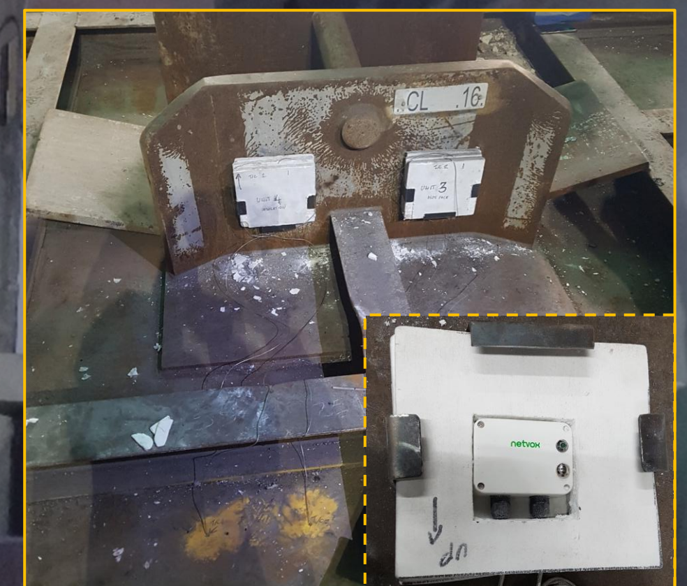
Figure 3: Two LoRaWAN units are installed on a caster lid. Inset Image: A unit encased in insulation board.
